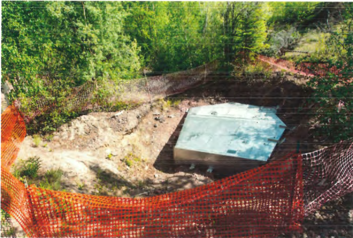
Figure 5: Stainless Steel Cap Installed Over Vertical Opening at the Cinch/Cenex Mine Site in Northern Saskatchewan
